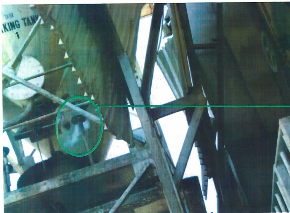
Fig 28 leakage from steam Pipeline
