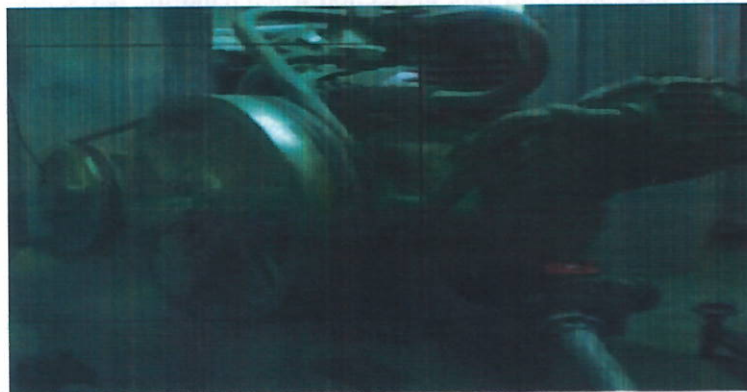
Fig 29 Unguarded drive of a reciprocating compressor
