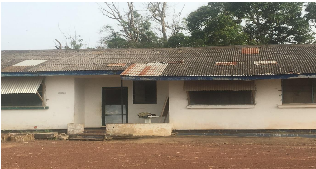
Figure 4: part of staff house to be rehabilitated with asbestos roof sheets.
