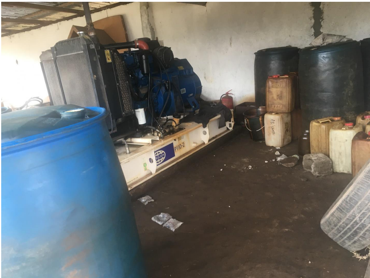
Figure 9: Spillage effect inside a standby power generator being operated in the PMU, MoA
